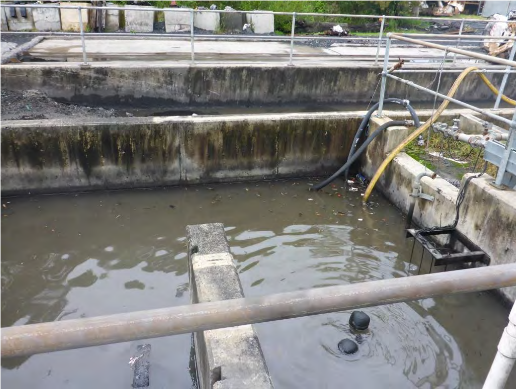
Photo 7 The Oily water separator worked effectively during the audit period
