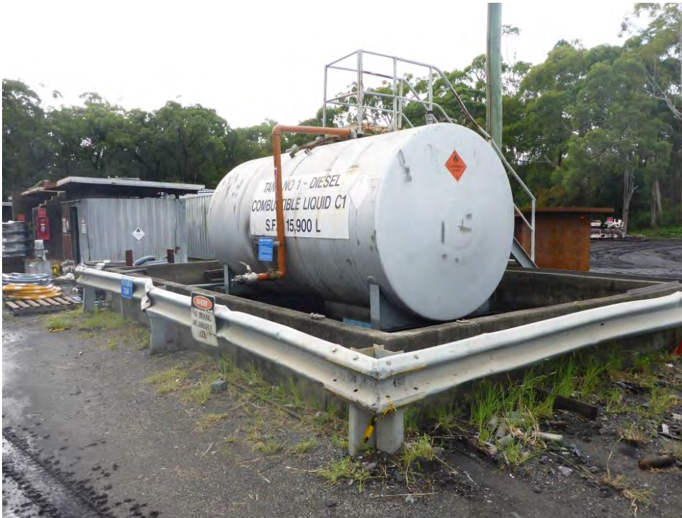
Photo 5 Diesel Tank stored within Bund
